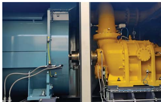
Photo 3. Basis of BCS-2 – screw compressor with electric engine
