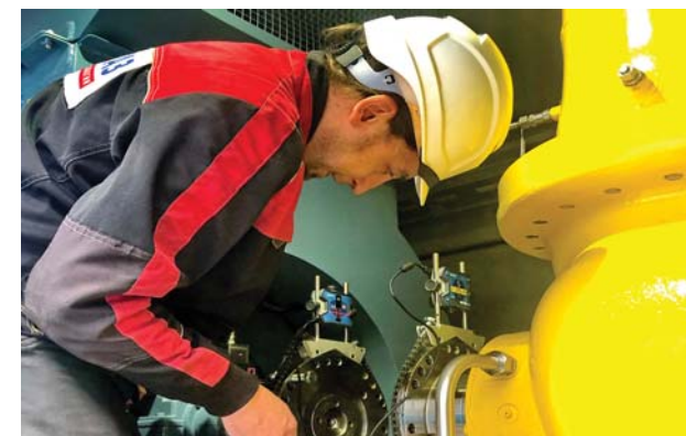
Photo 8. Comprehensive commissioning of the equipment was fulfilled by the ServicENER GAS experts
