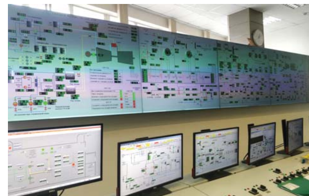
Photo 7. Both compressor stations are controlled from the upper level – from the CCGT control room
