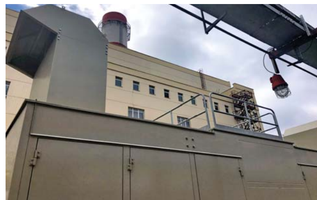
Photo 2. New booster compressor station for fuel gas from ENER GAS
